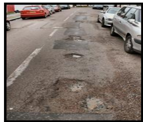
Figure 3.15.3e – Surface begins to pothole between areas already patched.
