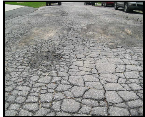
Figure 3.15.3g – Whole road surface needs replaced.
