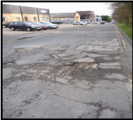
Figure 3.15.3f – Defects become more widespread.
