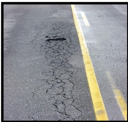
Figure 3.15.3d – Surface begins to pothole and rut.
